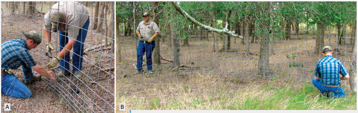
Figure 6. An extra pair of hands is helpful when attaching panels. One person holds the panels in place while the other secures them (A). After all the panels are secured, pull them to their desired location (B) to form a circle or teardrop shape.
