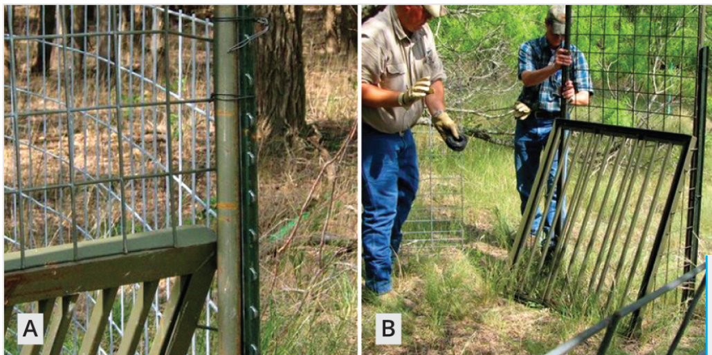
Figure 4. Use steel T-posts to secure a head gate (A). Make sure the head gate fits snugly against the T-posts using a doubled strand of baling wire (B).
